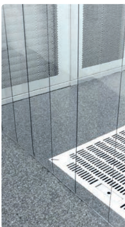
► The end of aisle containment solution consists of a "goal-post" frame housing antistatic curtain to prevent the mixing of hot and cold air.
